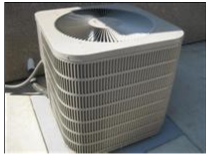
11.11 Picture 3 Compressor short cycles
